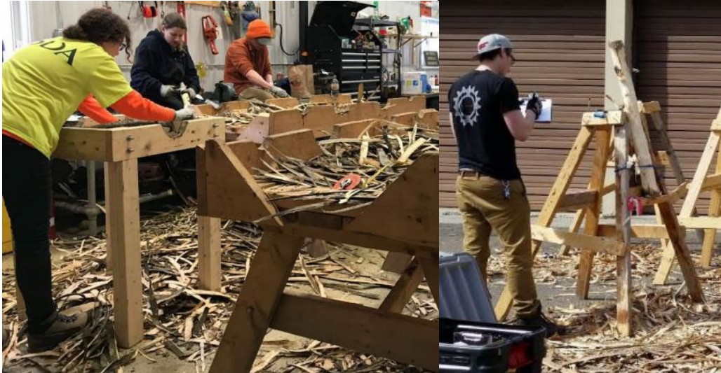
(Left) A peeling table. (Right) A peeling stand.
